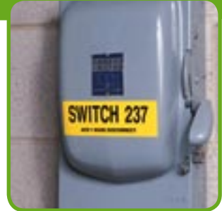
Panel & Switch I.D.
